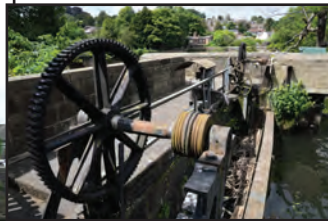
Water system machinery.
